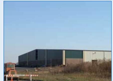
Construction of Amerhart's new facility in West Salem's Lakeview Business Park is currently underway by Wieser Brothers
