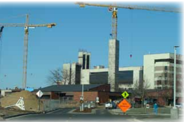
Construction of Gundersen Lutheran's new 400,000 square feet hospital began in early 2011. The new hospital will be built in phases over the next eight years.
