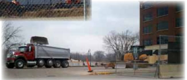
Viterbo University and the La Crosse Community Theatre recently teamed up to break ground on the La Crosse Performing Art Center. The 30,000 square feet, $9.6 million theater on the Mississippi River will seat 450.
