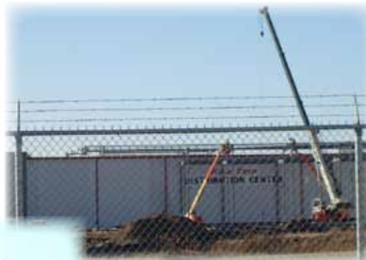
Kwik Trip continues to grow its corporate presence in La Crosse with a large addition to its distribution center.
