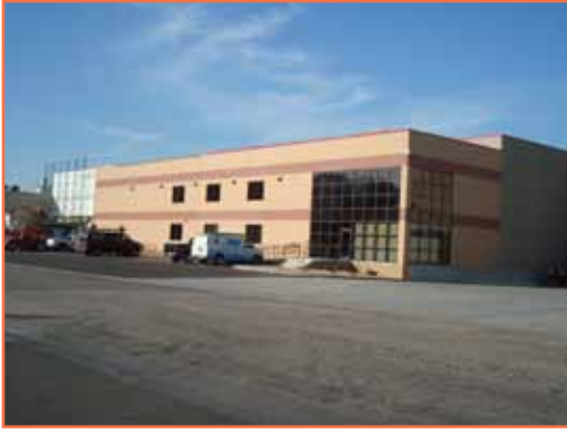
Kwik Trip's bakery addition is nearing completion. This project, estimated at $30 million, has doubled the size of the bakery and will add over 100 jobs.
