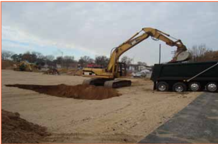
November 2010 - Trane Company's contractors remove the underground environmental contamination leading to a “clean site”.
