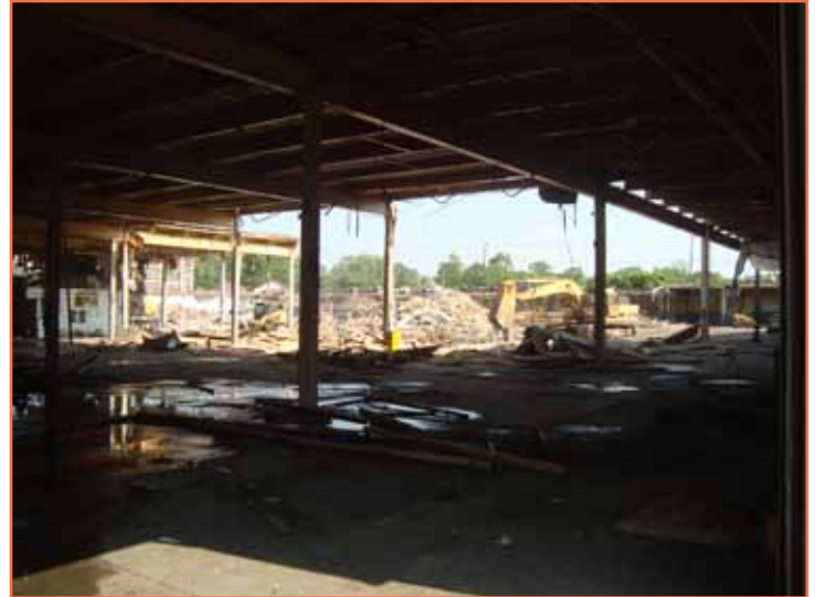
May 2010 - The roof and much of the inside components of the building were removed before the exterior walls, allowing nearly 85% of the building materials to be recycled or reused.
