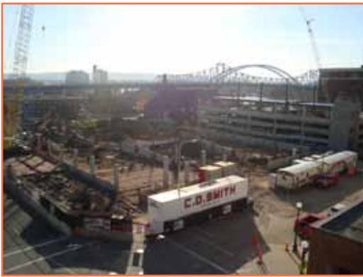
Construction of the $19 million Riverside Center III and the $12.5 million parking ramp began this summer. When complete, the facility is expected to house 700 employees.
