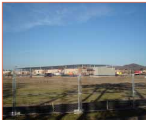
Construction of the new Gander Mountain store in Crossing Meadows in Onalaska began recently.
