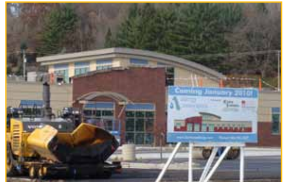
Construction continues on the new facility for Allergy Associates of La Crosse on Midwest Drive in Onalaska
