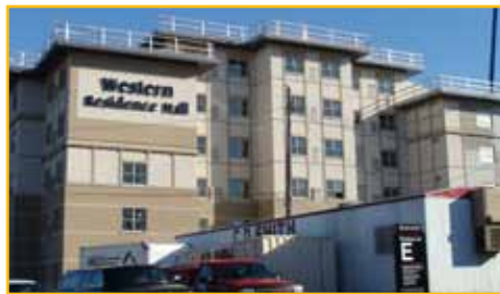
Construction of a new $10 million, 200 bed Residence Hall on Western's campus continues
