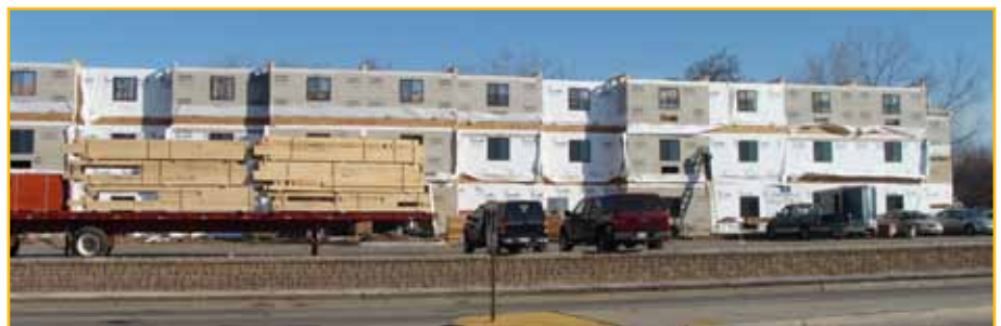
Phase II of 3 Rivers Plaza recently got underway with construction of the 92 room Candlewood Suites
