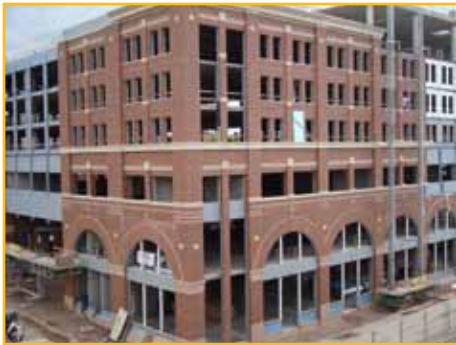
Construction of the Grand River Station transit center continues. Upon completion of the transit center, construction of housing units focused on expanding the arts community in Downtown La Crosse will begin above
